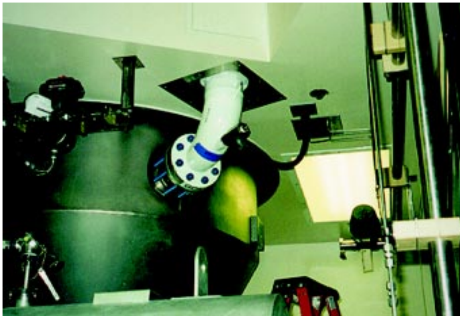
Explosion suppression system installed on a spray dryer.
