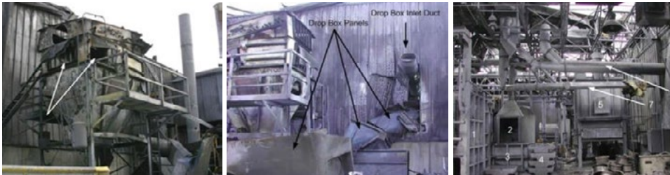
Figure 3: Damage after an aluminum dust deflagration: dust collector (left picture), drop box (center picture) and interior of the facility (right picture) (Chemical Safety Board, 2005)
